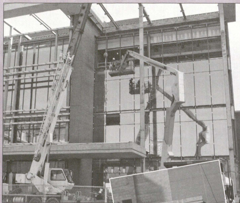
Workers install glass into the curtain-wall frames on the front of the Moakley building, along Harrison Avenue.
