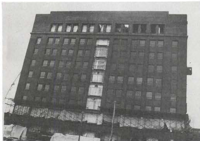
Work on the Center for Advanced Biomedical Research, the first building being constructed in BioSquare, has reached an advanced stage. Interior petitions have been installed on many floors and the installation of laboratory and plumbing fixtures is under way.
