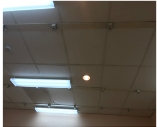
Ceiling fitted for suspension
