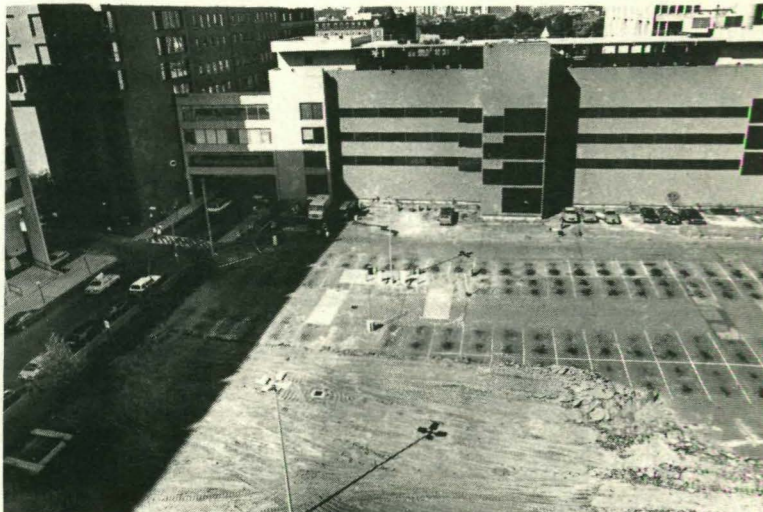
OUT WITH THE OLD: Parking Lot A on East Newton Street closes in preparation for the construction of the Hospital's Partial Replacement Project.
