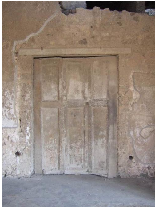
Figure 8. Preserved door partition attached to cubiculum 16 in the Villa of Mysteries in Pompeii. (Source: Pompeii in Pictures )
